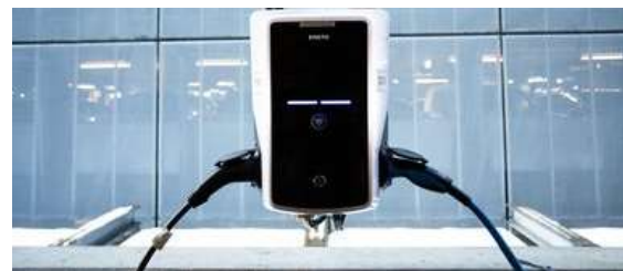
Charging possibilities in the parking garages
